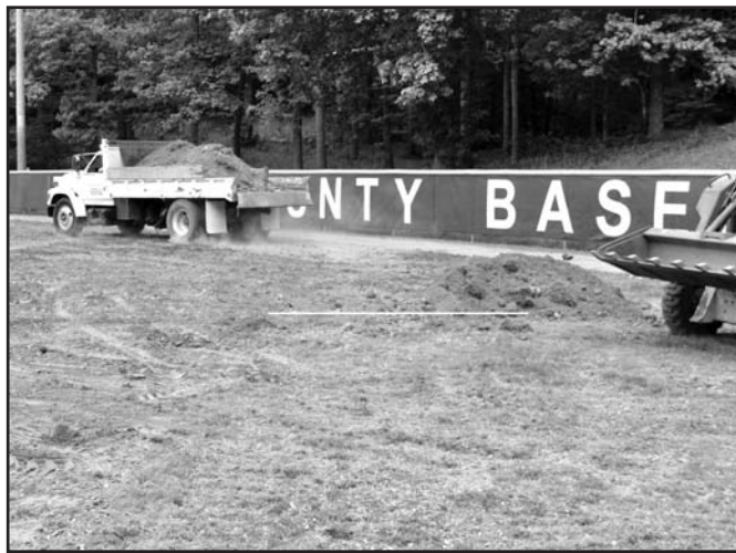
Photo by Mark Novak Drain construction at the Towns County Baseball Field.
